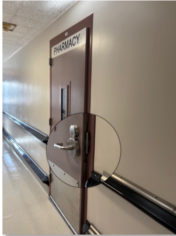
Photo 19. Main pharmacy door found unsecured and unlocked. Photographed on 5-13-2026.
