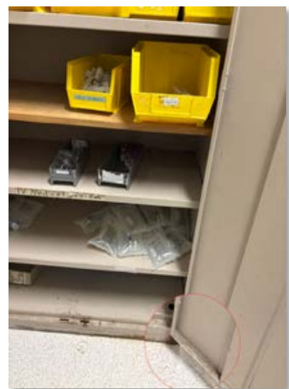
Photo 5. Unclean supply cabinet. Photographed 4-6-2026.
