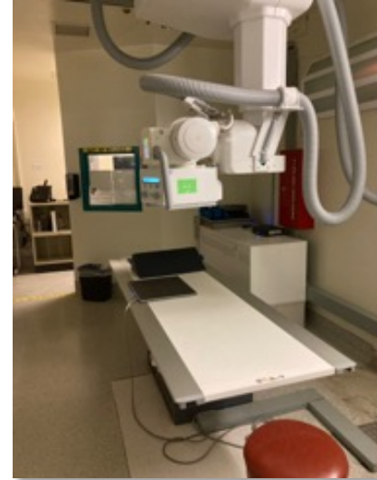
Photo 2. Radiology room equipment. Photographed on 4-22-2026.
