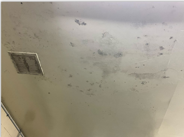
Photo 5. Mold or mildew on ceiling at CSP-Sacramento. Source: OIG audit staff.
