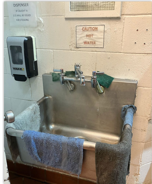
Photo 8. Dirty towels drying in hand sinks at Richard J. Donovan Correctional Facility. Source: OIG audit staff.
