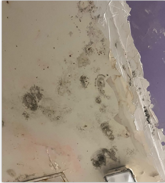
Photo 13. Mold or mildew on ceiling in kitchen at CSP-Corcoran. Source: OIG audit staff.
