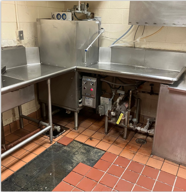
Photo 3. Missing tile and dripping hose lines in kitchen at CSP-Sacramento. Source: OIG audit staff.
