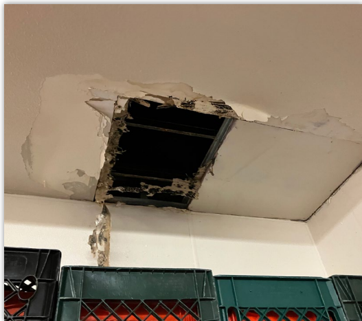
Photo 14. Hole in scullery ceiling at CSP-Corcoran. Source: OIG audit staff.
