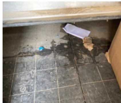
Photo 9. Floor was found soiled. Photographed 2-3-2026.
