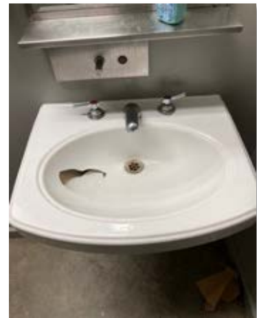
Photo 9. Sink in disrepair. Photographed 1-5-2026.
