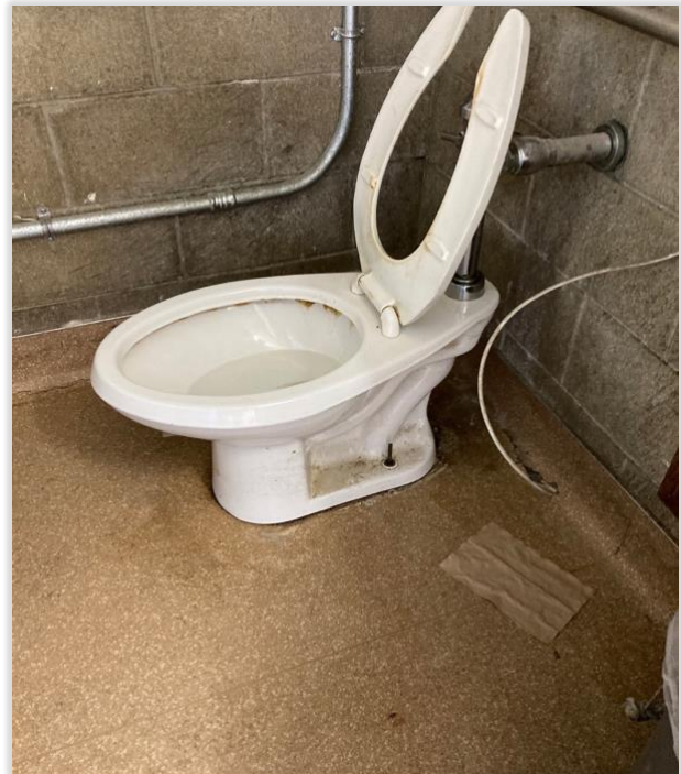
Photo 6. Staff restroom was unsanitary (photographed on 8-2-23).
